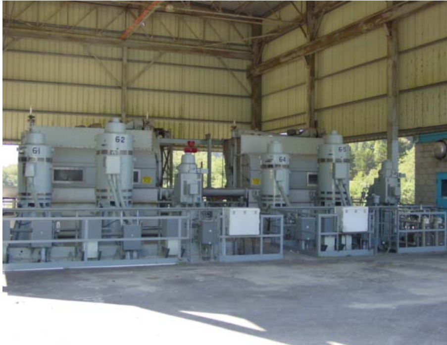
Electric-Driven Pump Motors at Direct Diversion Facility
