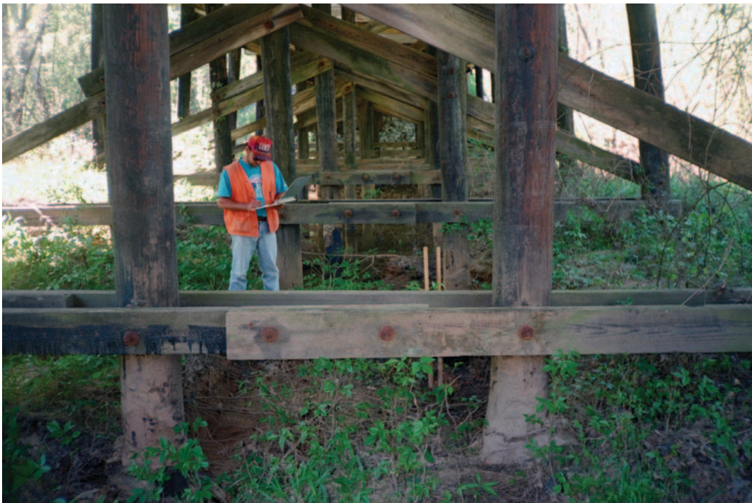
Figure 98. Clear-water contraction scour on the right overbank as viewed from the left at Structure 367008100200 on Road S-81, crossing the Enoree River in Newberry County, South Carolina. (Photograph by the South Carolina District, U.S. Geological Survey, April 7, 1997.)
