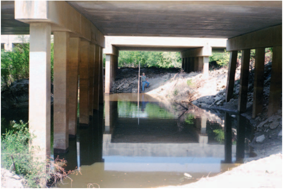
Figure 81. Scour hole at left abutment viewed from downstream at Structure 264000920500 on S.C. Route 9, crossing the Waccamaw River in Horry County, South Carolina. (Photograph by the South Carolina District, U.S. Geological Survey, June 2000.)
