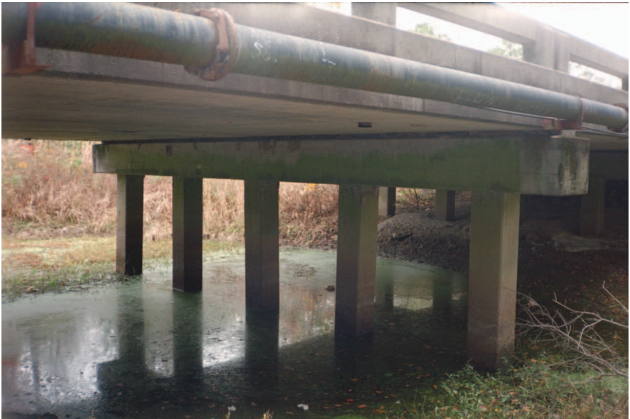
Figure 21. Concrete pile bent at Structure 182007800200 on U.S. Route 78, crossing Polk Swamp in Dorchester County, South Carolina. (Photograph by the South Carolina District, U.S. Geological Survey, November 26, 1996.)
