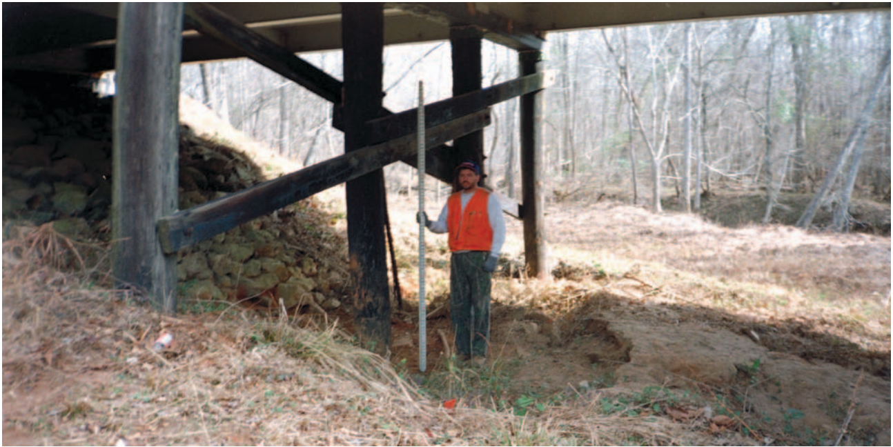
Figure 19. Timber pile bent at Structure 194023000500 on S.C. Route 230, crossing Horne Creek in Edgefield County, South Carolina. (Photograph by the South Carolina District, U.S. Geological Survey, February 6, 1997.)
