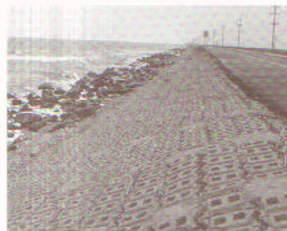
The "hard structure" approach to protecting a road from the sea on Cape May, New Jersey.
