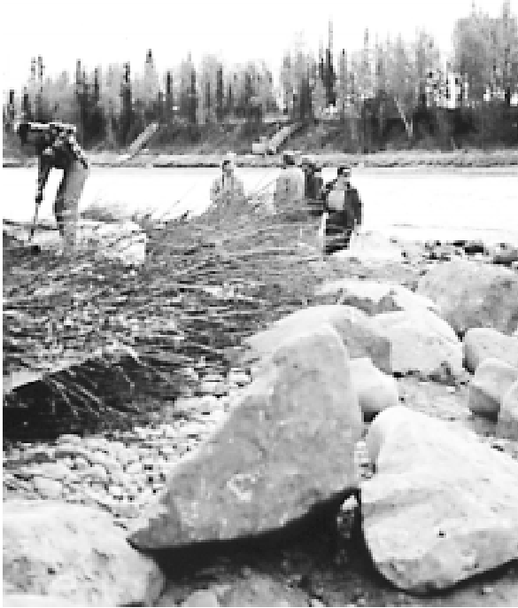
Bioengineering techniques, such as the willows shown here, were used for bank stabilization along the Kenai River, AK.
