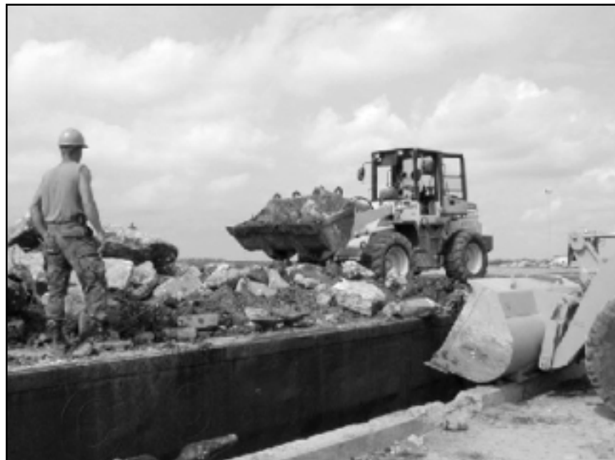
Debris being moved to form Charleston Air Force Base Offshore Reef Project.
