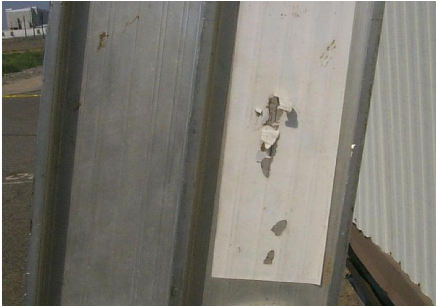
Exhibit 2-3, Faded label on ladder used at MO-392, south wall.
