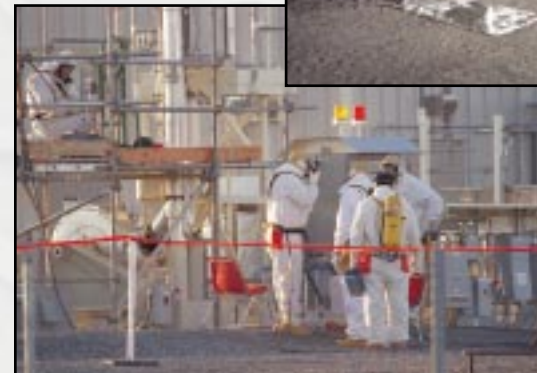
Top: Screen is installed in an underground single-shell tank so that radioactive liquid wastes can be pumped out. Bottom: Workers practice Tank C-106 sluicing process.
