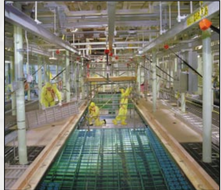
K West Basin floor grating is removed to make way for fuel retrieval system installation, now under way.
