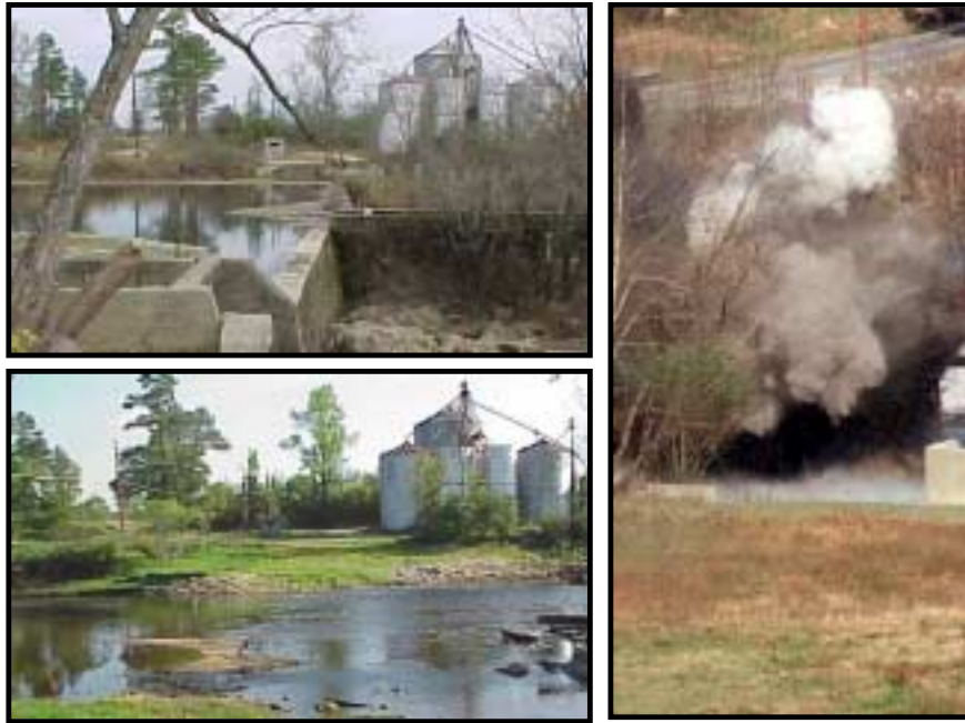
Photo 15. Rains Mill Dam (top left before demolition), Explosive Removal on December 1, 1999 (right), and in the Spring After Demolition (bottom left)
