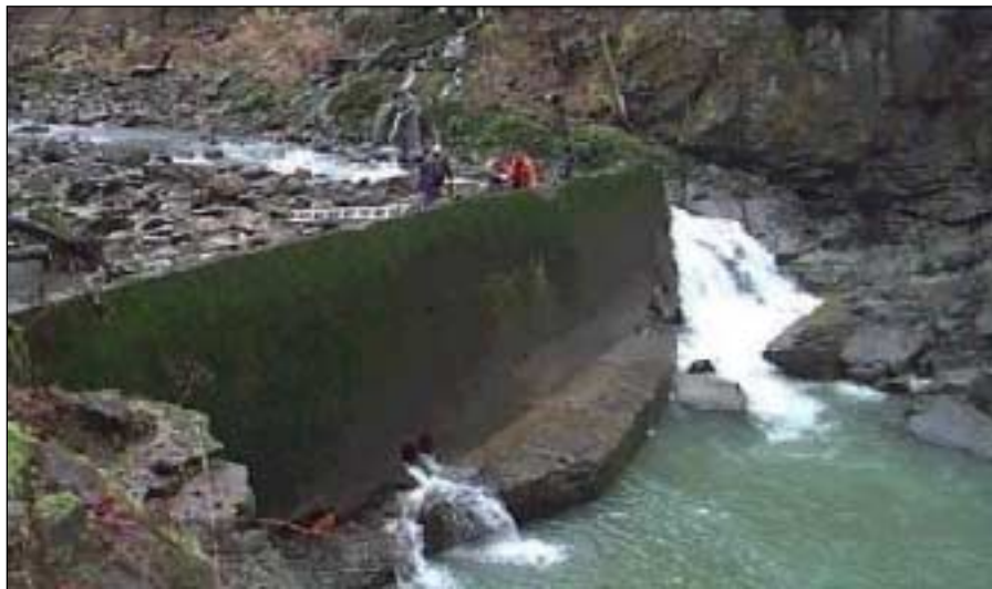
Photo 1. The LaGrande Construction Dam on the Nisqually River, Removal Under the SFO Program in the Spring 2000
