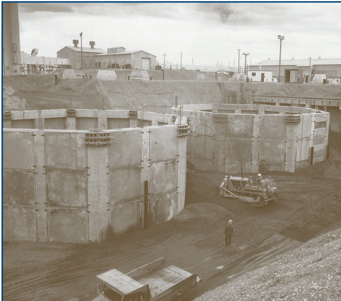
Figure 20. The INTEC tank farm, shown under construction during the 1950s, is the principal source of contamination at the INTEC. The tanks themselves are not known to have leaked.
