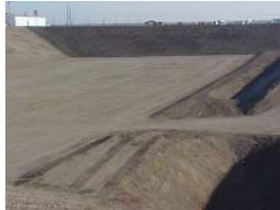
Construction of the INEEL CERCLA Disposal Facility continues. A public workshop on the progress of the engineered landfill will be held on May 20 at the Ameritel Inn in Idaho Falls.
