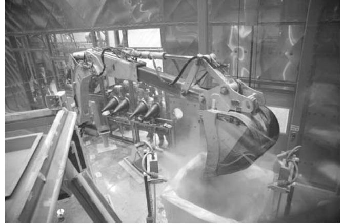
Workers excavate overburden soil using a backhoe. The backhoe arm is sealed within a retrieval confinement structure.
