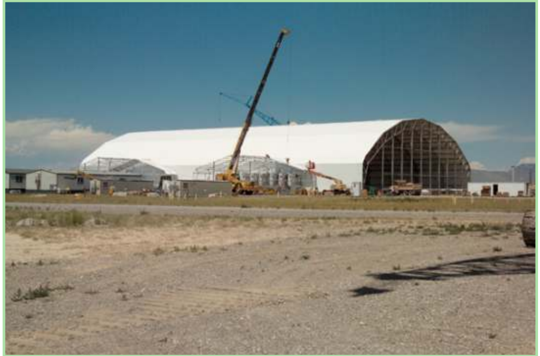
A portion of the transuranic waste buried in the Subsurface Disposal Area will be excavated inside a retrieval structure (above).
