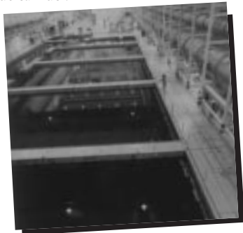
Spent nuclear fuel currently in underground storage basins at the Idaho Nuclear Technology and Engineering Center must be removed from the state by 2035.
