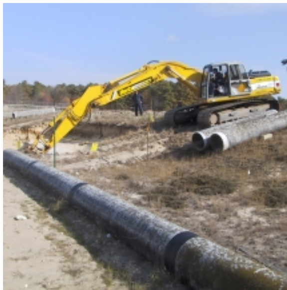
In November 2002, workers at the Sewage Treatment Plant remove sediment containing elevated levels of mercury
