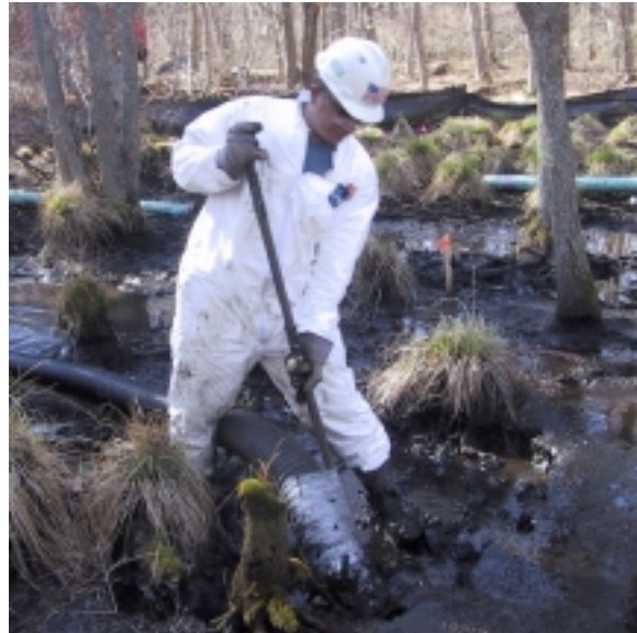
In April 2002, worker frees sediment leaving wetland vegetation undisturbed during Peconic River pilot-study project
