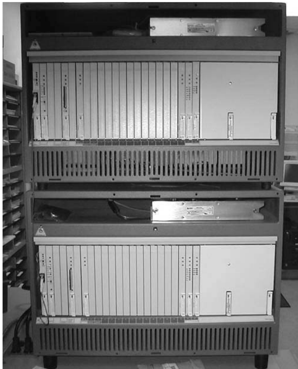
Left: New Definity Prologix G3si as installed at Culpeper and Arlington sites.
