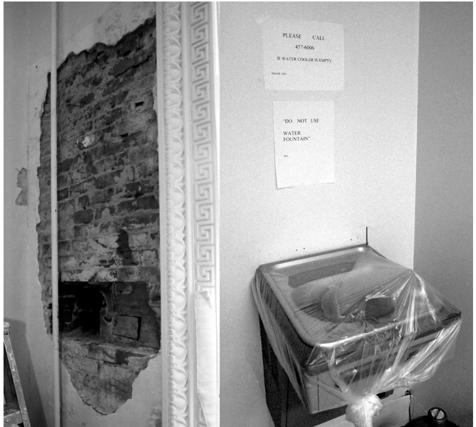
Figure 6: Water Damage in EEOB in Washington, D.C., and Covered Water Fountain with Posted Warning Against Drinking the Water in FOB 3, Suitland, Md.
