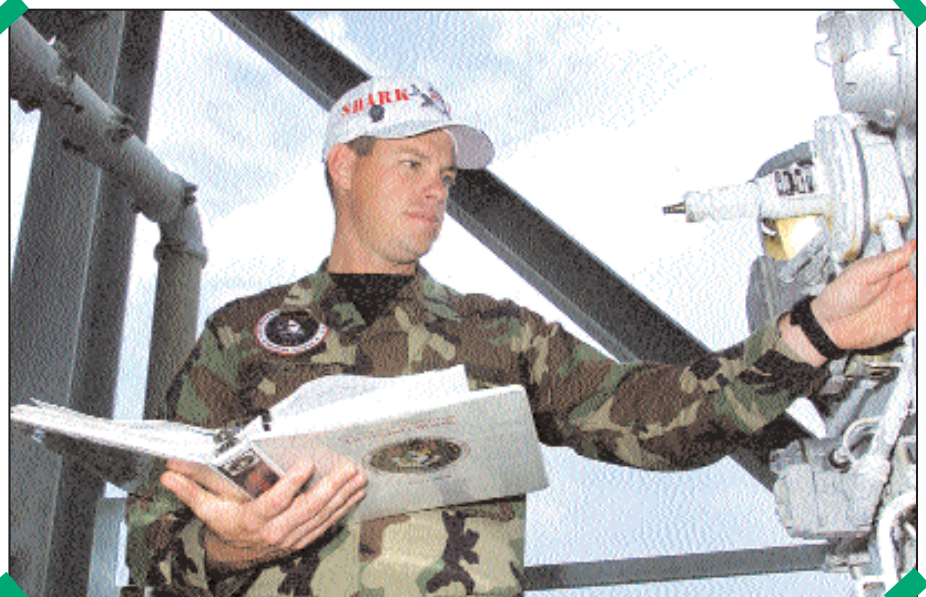
Today's 14th AF plays an integral role in providing victory to the warfighter through space. Tech. Sgt. Philip Lemaitre, maintenance controller at the 3rd Space Launch Squadron, inspects the controller panel that opens the environmental shelter's door at Space Launch Complex 40 at Cape Canaveral Air Force Station. (Photo by Senior Airman Anne McCormick)
