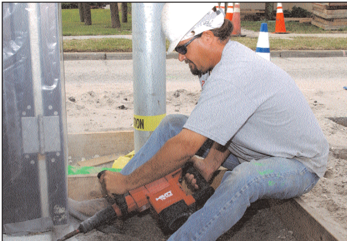
Shannon Light, a carpenter contracted to work on the new Patrick Air Force Base Main Gate, drills a hole through concrete to run electrical wires. All construction plans go through the 45th CES engineering office.
