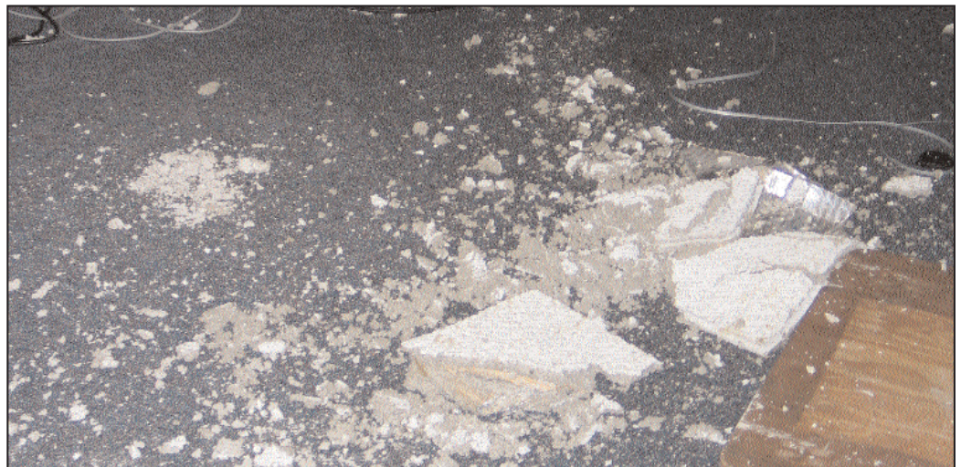
Pieces of ceiling tile and water cover the floor of Education Center classrooms due to the hurricane.
