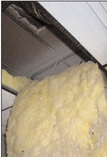
Insulation hangs where the weight of the water was too much for ceiling tiles. Two wings of the Education Center were badly damaged.
