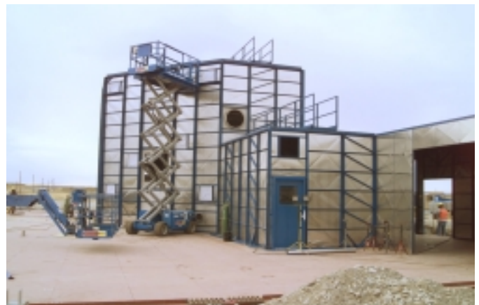
Construction of the retrieval confinement structure at Pit 9 is nearing completion. Construction on the weather enclosure is underway.
