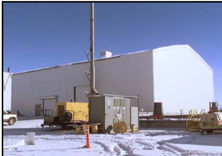
Construction of the weather enclosure at the glovebox excavator project was completed in November 2002.
