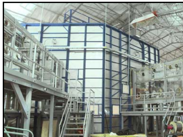
Construction continues on the Glovebox Excavator Method project. This photo shows the inside of the weather enclosure.
