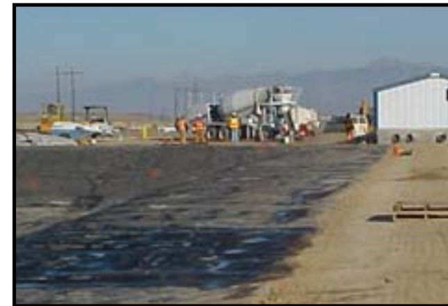
Work is progressing on support buildings for the completed disposal cell and evaporation ponds at the INEEL CERCLA Disposal Facility complex near the Idaho Nuclear Technology and Engineering Center.
