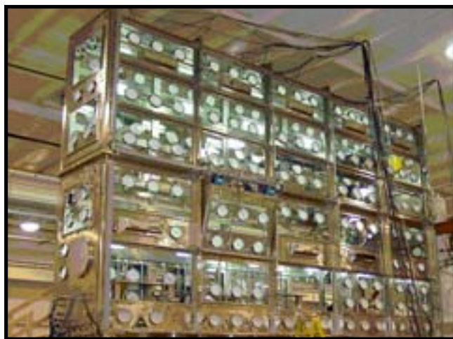
A series of gloveboxes are in place at the Advanced Mixed Waste Treatment Facility. The project is working towards startup by the March 31, 2003 commitment with the state of Idaho.
