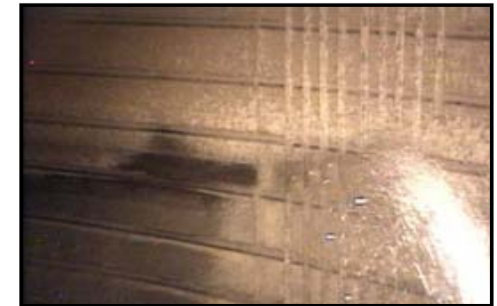
Tank cleaning is underway at the tank farm. To date, cleaning has been very effective on removing the materials from the tanks.
