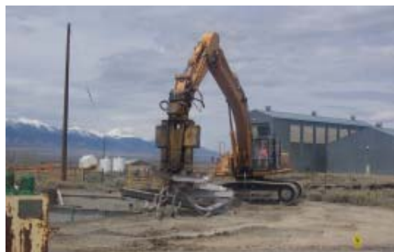
Significant progress is being made in eliminating excess buildings and structures at Test Area North. This year, 68,000 square feet has been removed.
