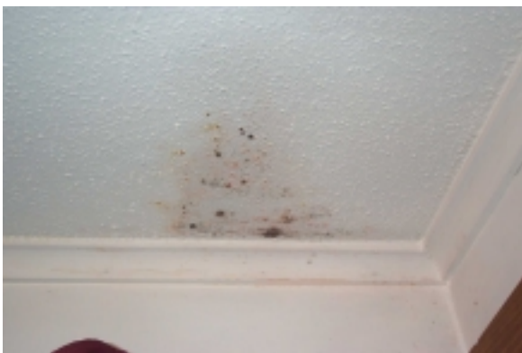
Discoloration (mold?) at ceiling under soffit vent.
