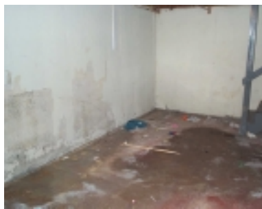
Basement before refinishing, with some water entry.
