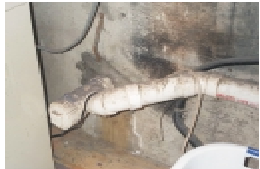
Unintended water entry by sewer line.
