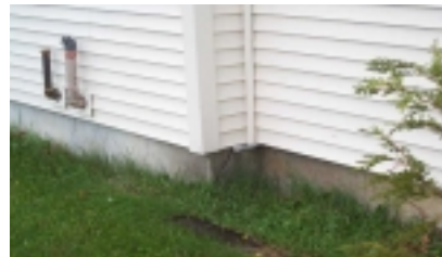
Foundation crack that could lead to water damage in basement. This type of damage can hide behind walls in finished basements.
