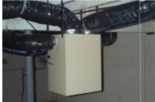
In winter, heat recovery ventilators can be used to increase the amount of ventilation without losing heat.
