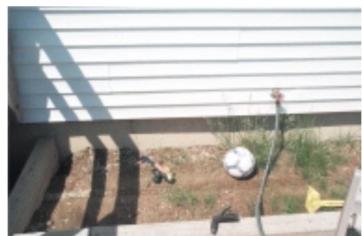
...outside planter with unintended drainage down outside basement wall.
