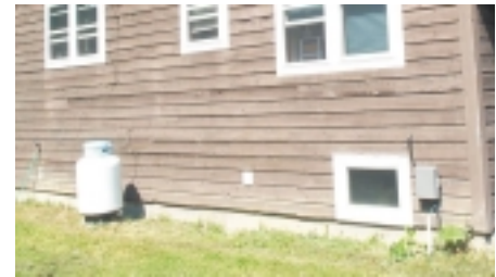
Depression in soil at the sewer pipe may lead to water entry.
