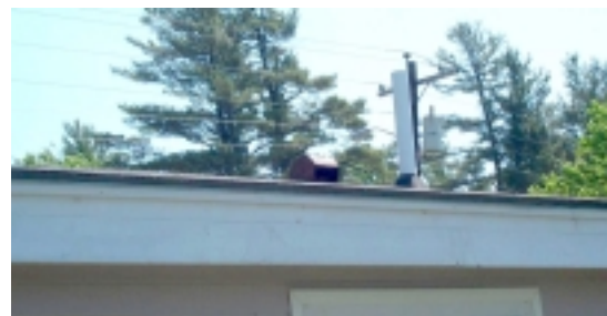
Site of water entry into fan above scoop that faces prevailing winds.
