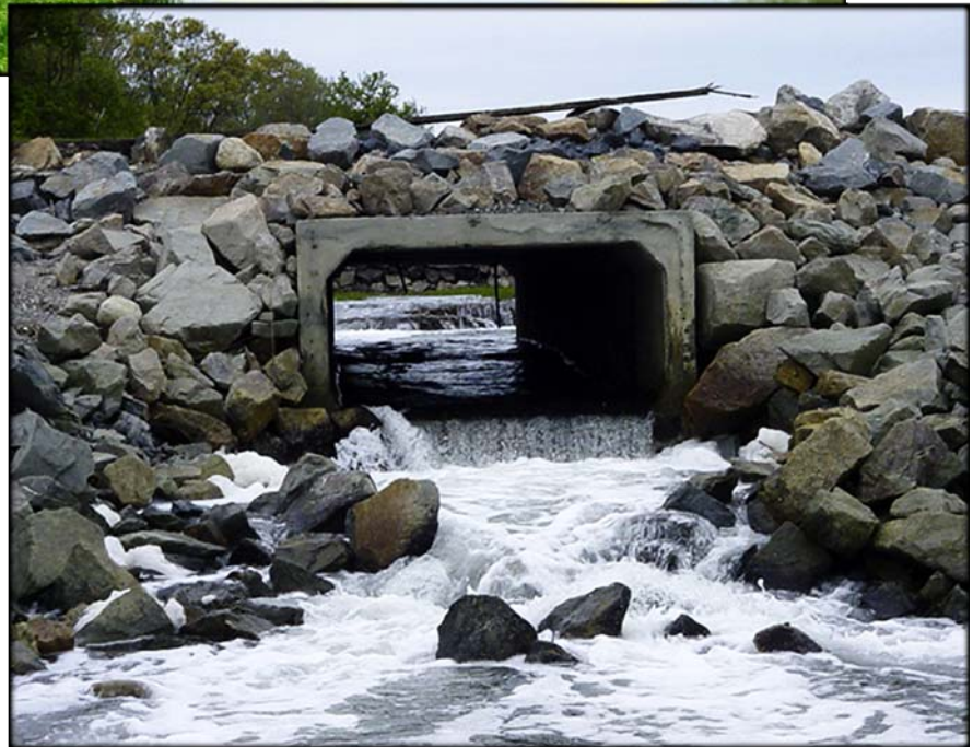
Tidal flow created through the installation of culverts, restoring Damde Meadows to a natural salt marsh, Hingham, MA.
