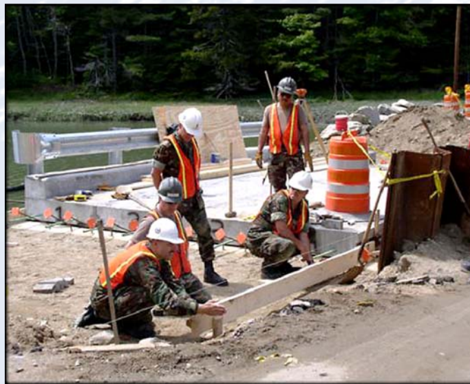
The Navy Seabees (Innovative Readiness Training program) from NMCB-27 provided equipment and labor to build the bridge to restore tidal flow to Dingley Island, ME.
