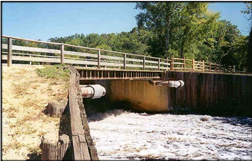
A fish ladder installed as part of the Batsto River Fishway Restoration Project in New Jersey.
