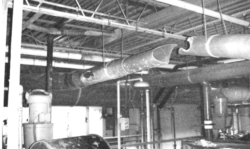
Figure 5. Large fracture of 10-inch branch duct above mezzanine 2 production area.
