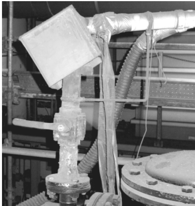
Figure A-1. Kestner unit exhaust ventilation.
