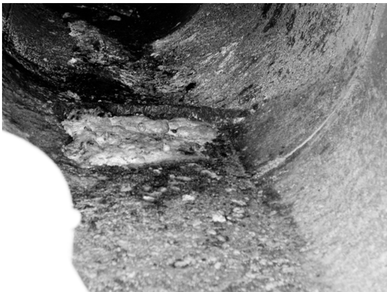
Figure 10. Solid deposits in main header duct.
