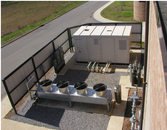
United Technologies fuel cell installed at the NTRC provides building power and temperature control.
