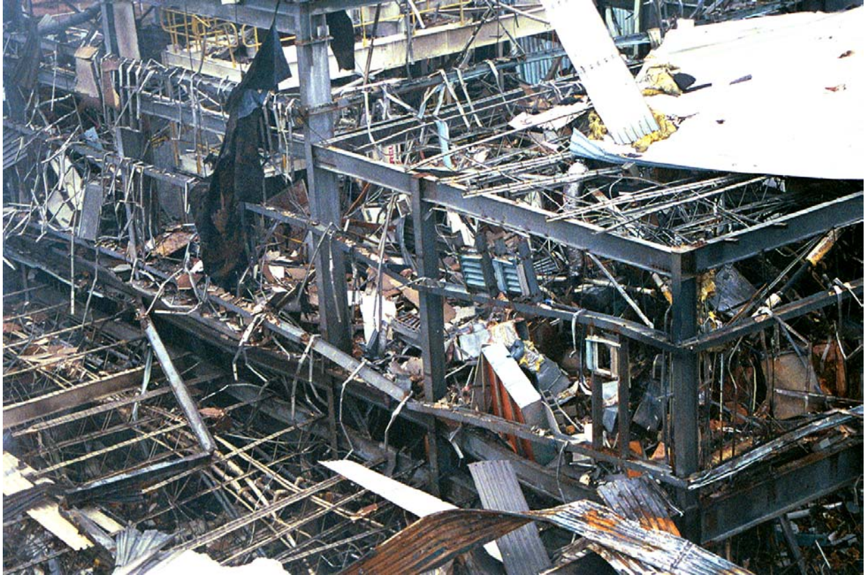
Figure B-3. Southwest wall of compounding area deflected outward.
