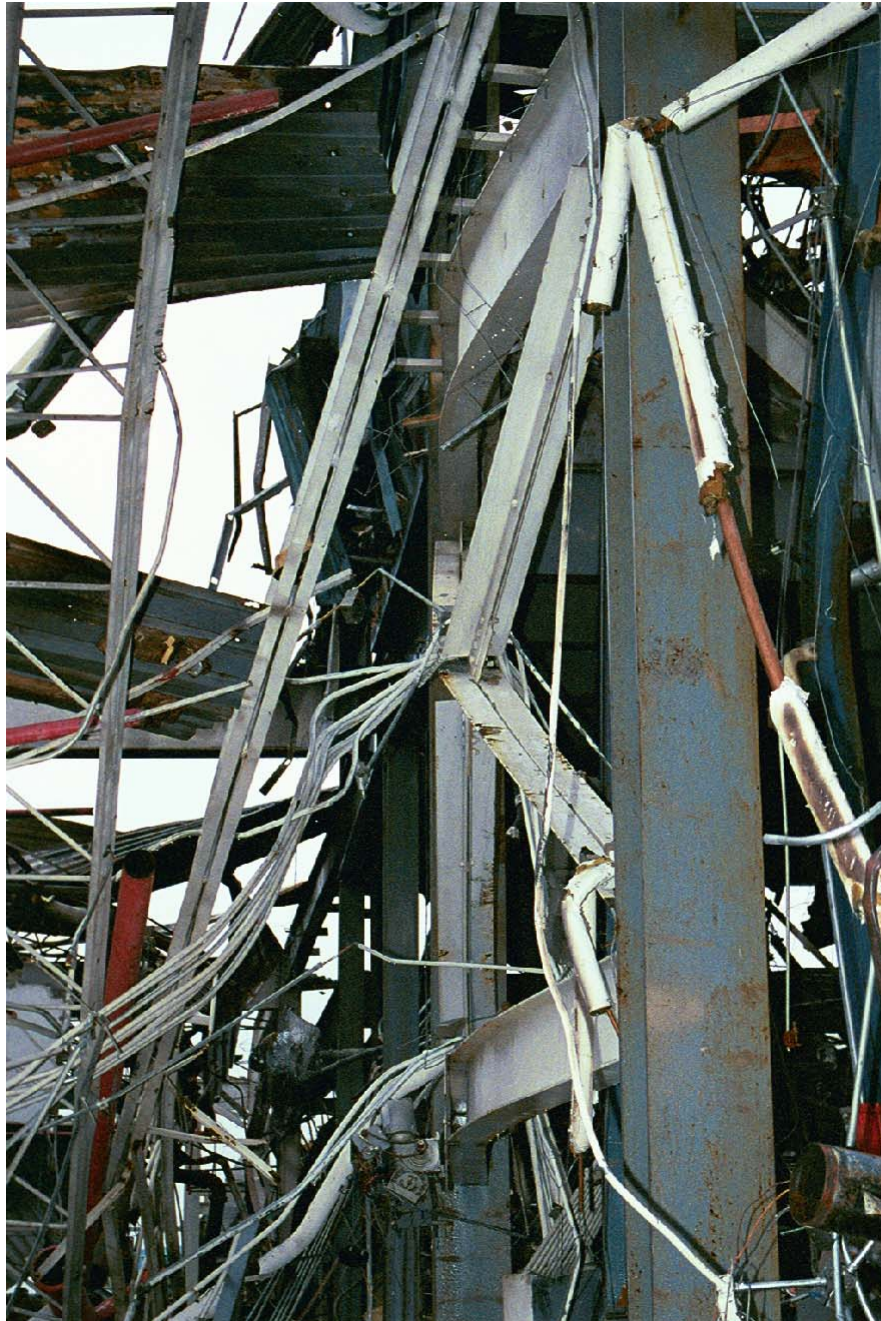
Figure B-1. Beam and cross bracing deflected southeastward toward warehouse.
