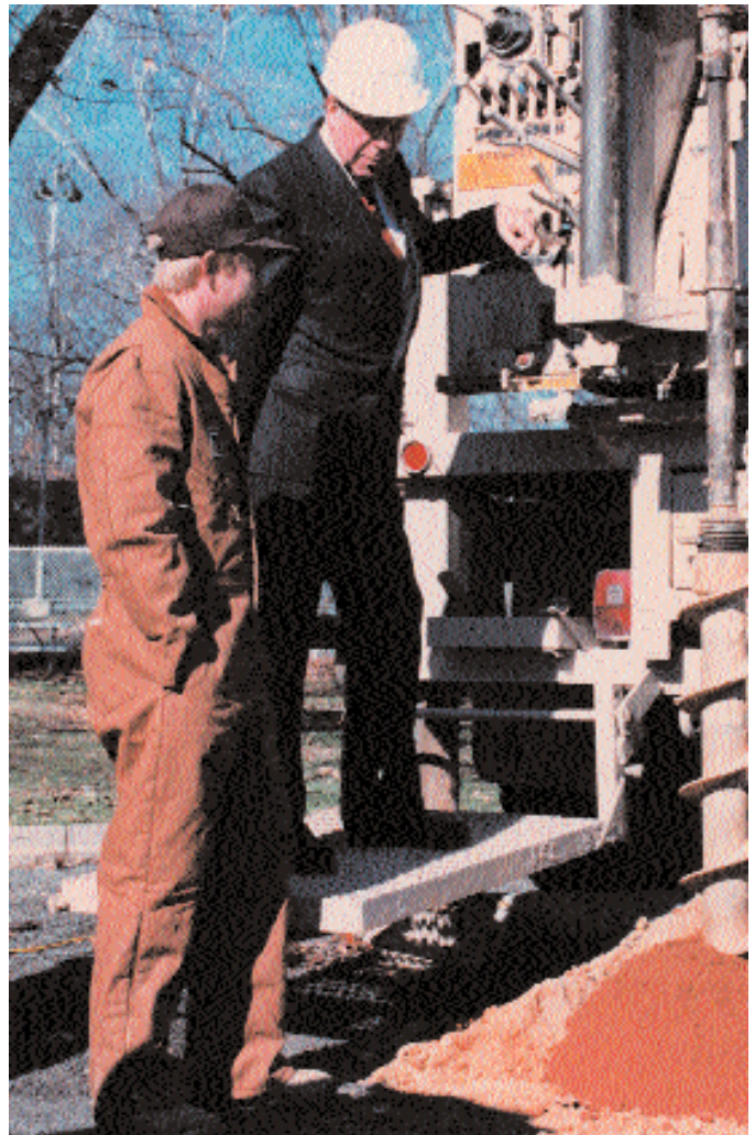
Secretary Shultz observes core sample drilling at Arlington Hall during a visit to the construction site in November 1988.
