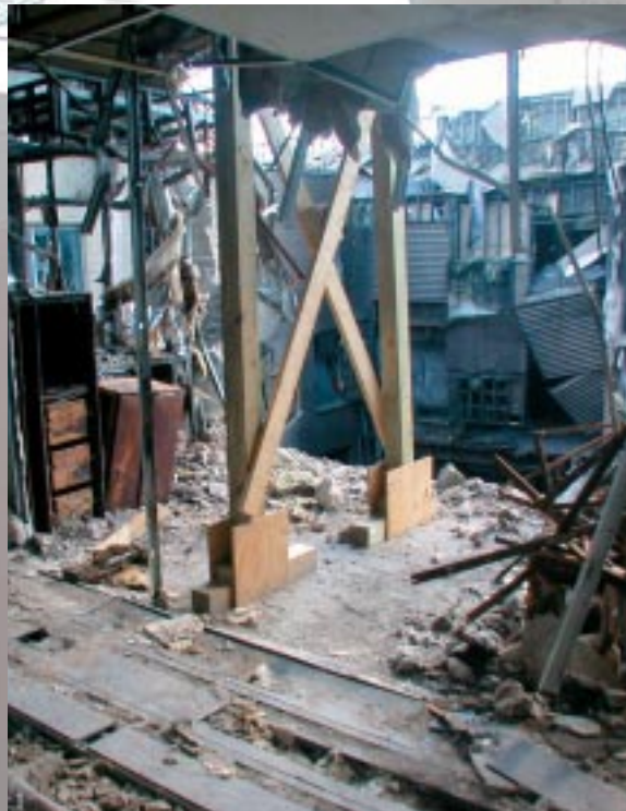
Wooden trusses support the remains of one office.
