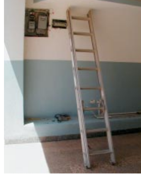
Aluminum ladder at an electrical box in a residence is set at the proper angle.
