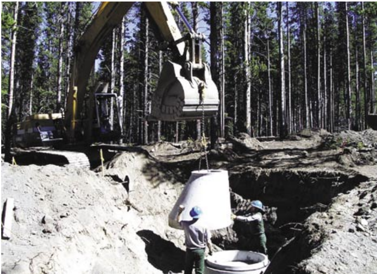
Yellowstone National Park (MT/WY/ID) is replacing failing sewer systems and installing new sewer lines throughout the park to protect park resources and better serve visitors.
