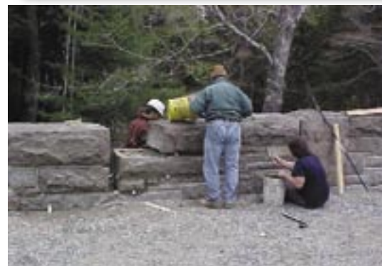
Acadia National Park (ME) is rehabilitating the surfaces, vistas, and bridges of the park's roads and carriage road system. The project will improve the safety, aesthetics, and accessibility of Acadia's road systems for the public.
