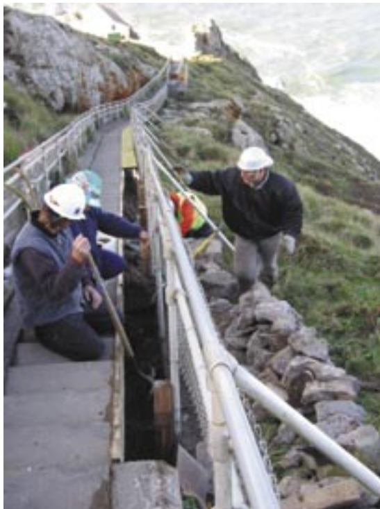
Point Reyes National Seashore (CA) is replacing old concrete steps and handrails to ensure safe visitor access to the historic Point Reyes Lighthouse Complex. The badly deteriorated 304-step stairway runs adjacent to the steep cliffs and is the only access to the main lighthouse.
