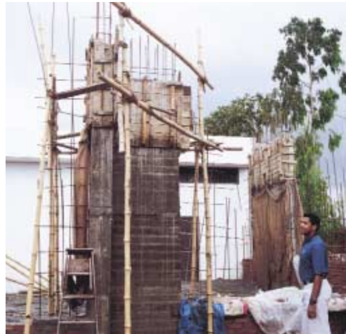
Facility manager Michael L. Jackson, right, inspects bamboo scaffolding at the commissary building site.
