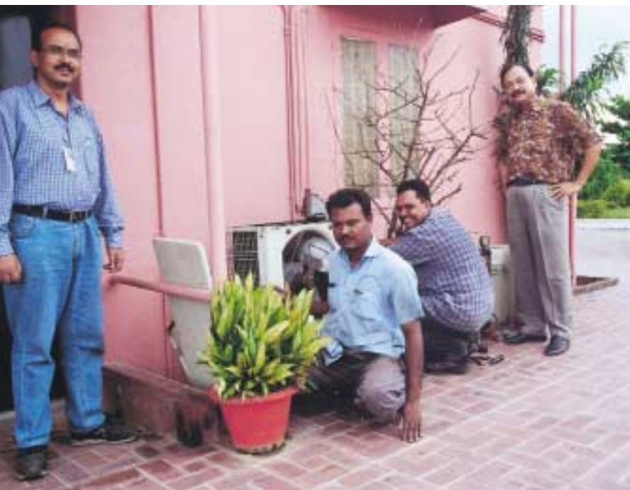
FSN staff repair an air conditioning unit at the general services office center. They are, from left, Naquibul Hossain, Auranzeb Bhuiyan, Alamgir Alam and Moshin Ahmed.
