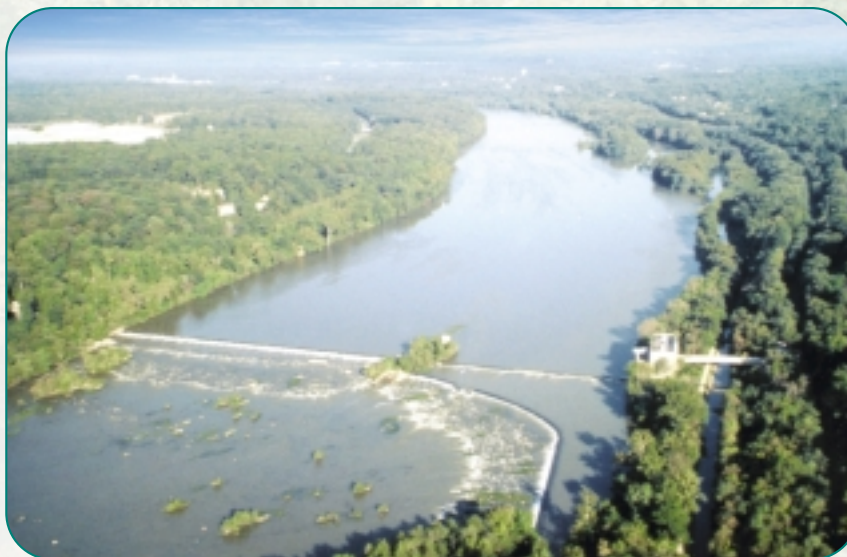
A Mid-Atlantic team constructed an innovative fishway at Little Falls Dam; MD
