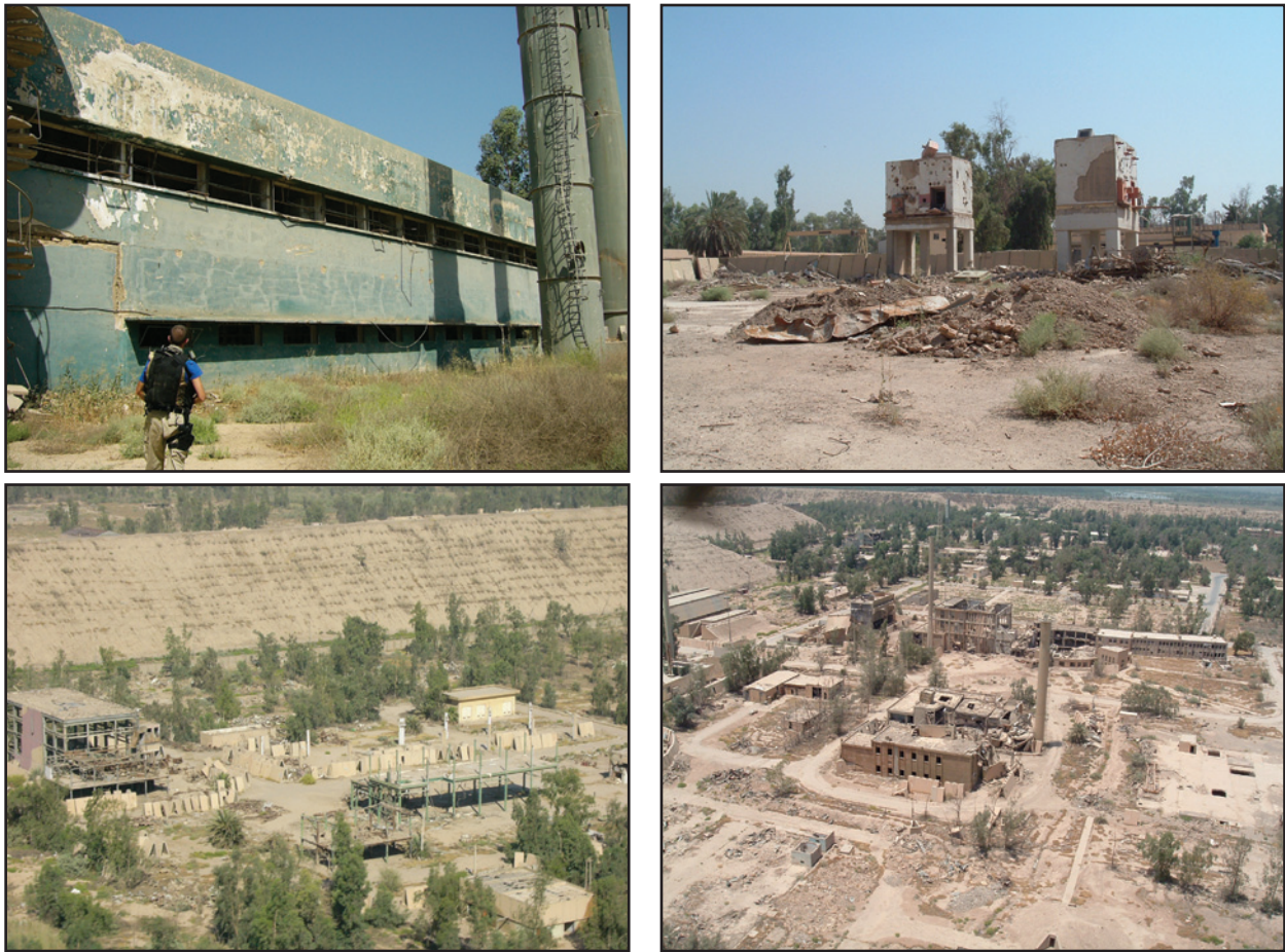
Figure 7. Tuwaitha Building 15 area (top left); Tuwaitha Building 15 area (top right); Tuwaitha Building 73 area destroyed (bottom left); Tuwaitha LAMA Facility (Building 22 destroyed) (bottom right).
