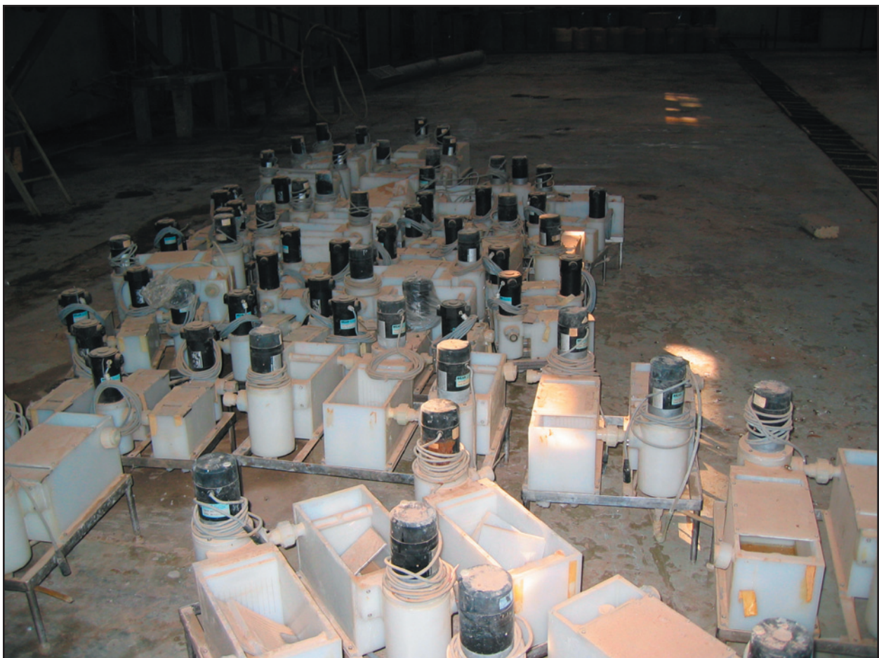
Figure 26. Mixer-settlers in storage at Ibn Sina (photo taken by ISG Team, December 2003).
