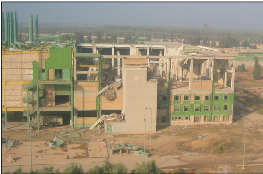
Figure 23. Destroyed Alpha-Enrichment building at Tarmiya (photo taken by ISG Team, December 2003).
