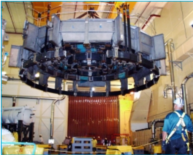
The disassembly of the Tokamak Fusion Test Reactor (TFTR) at PPPL progressed. On November 8, the umbrella structure and upper magnetic poloidal-field coils were lifted off the top of TFTR. Workers used the 110-ton capacity overhead bridge crane to make this 92-ton lift. Preparation for this critical lift began several months earlier. The structure and coils were removed as part of the disassembly of TFTR, which is expected to be completed by September, 2002.
