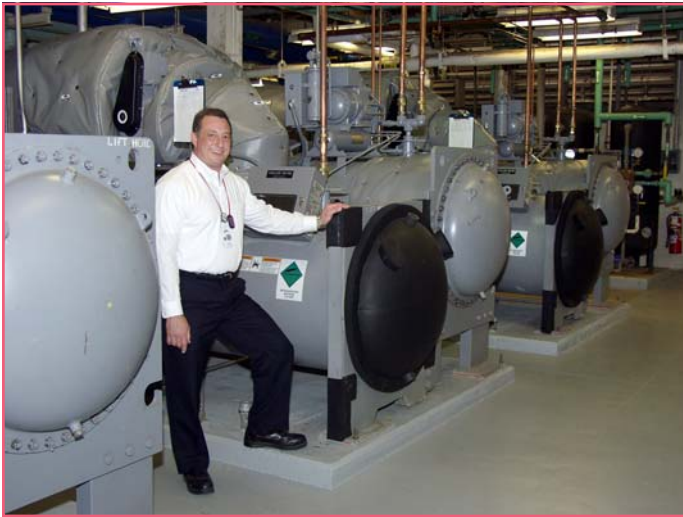
PPPL Engineer Henry Carnevale, who managed the chiller replacement project, is above with the new chillers. At right are the old chillers.
