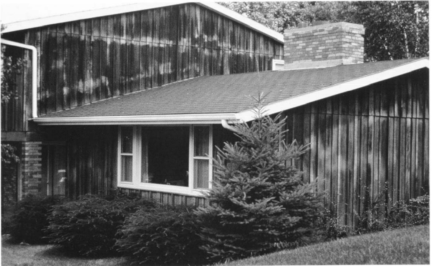
Figure 26---Lap marks formed by improper application of a semitransparent penetrating stain
