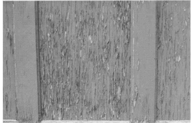
Figure 13—Early paint failure on plywood as a result of penetration of moisture into surface checks.
