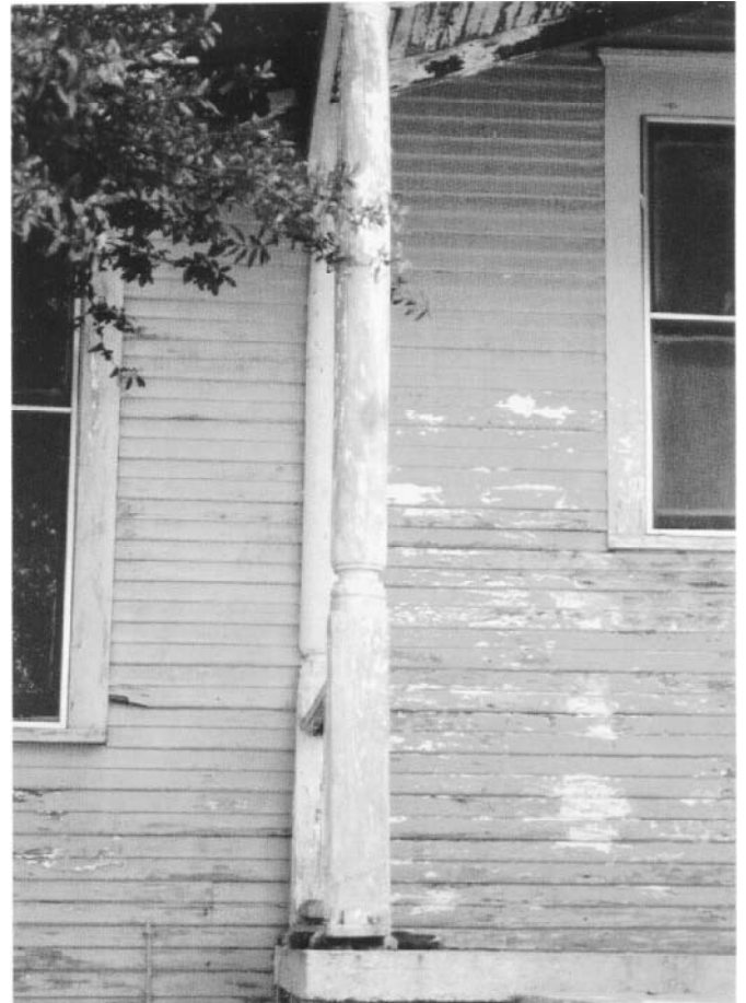
Figure 36---Paint can peel from wood when excessive moisture moves through the house wall. Some cross-grain cracking is also evident on this older house. (Photo courtesy of Southern Forest Products Association.)
