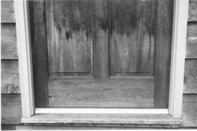
Figure 5-Rainwater splash on entrance door and siding. Rain water runs from the roof and wets the siding as it hits the concrete step.
