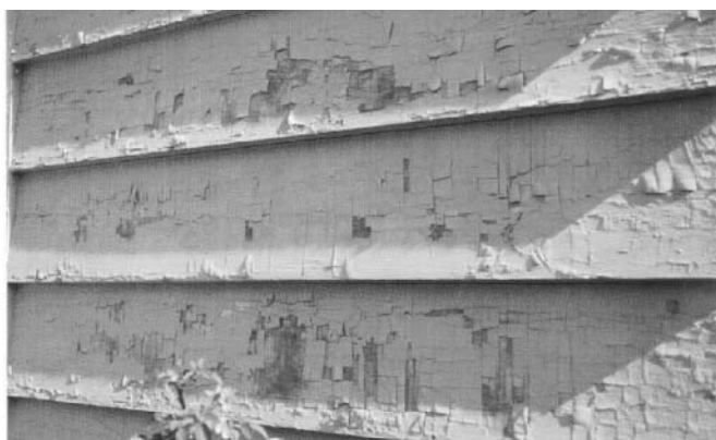
Figure 34---Cross-grain cracking results from an excessive buildup of paint.
