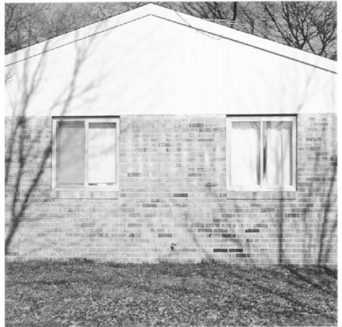
Figure 38—Chalking of paint. Some paints or stains chalk badly. Chalking can discolor a lower surface as the resin and pigment particles wash down.
