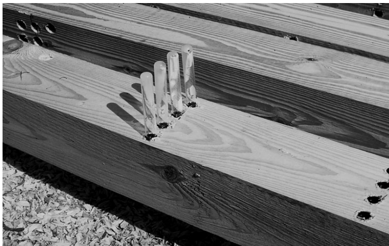
Borate preservatives applied through adsorption of the liquid in a series of drilled holes.
