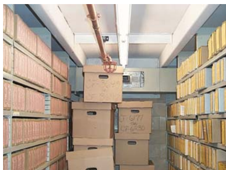
Stored materials prevent proper operation of fire sprinklers
