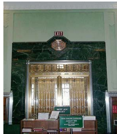
Conflicting Exit Signs for Doorway
