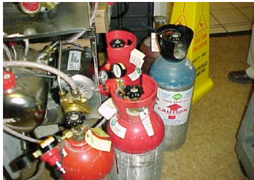
Unsecured Compressed Gas Cylinders
