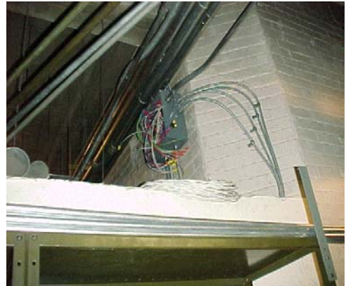
Electrical Junction Box with no Cover and Energized Wires
