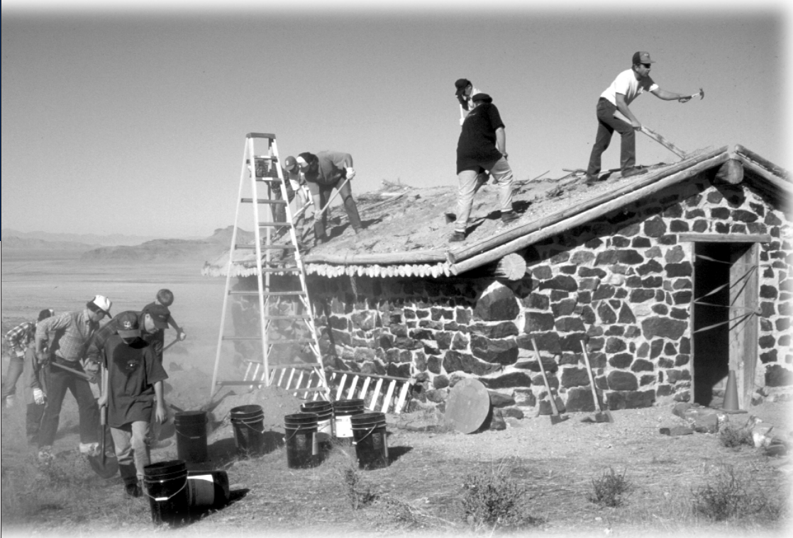
Volunteers repair the roof of a Pony Express Station to stabilize the historic structure in West Desert, Utah, and make it safer for visitors.
