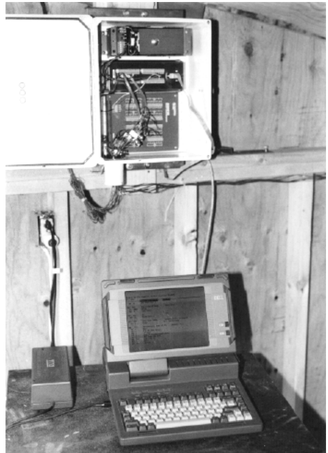
Figure 5—Set-up of datalogger–multiplexer, temporarily attached to downloadable, portable computer system. (M95 0057–21A)
