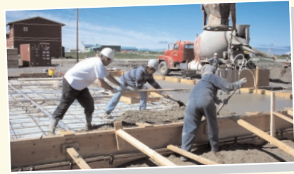
Local workers pour the foundation for the clinic's ambulance garage. USDA Rural Development provided funding for Unalakleet's new ambulance under the "Project Code Blue" program.
