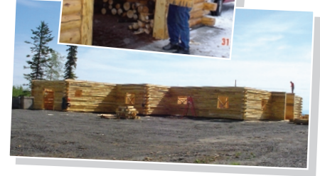
MINTO COMMUNITY HALL Minto Chief Andrew Jimmie cuts the ribbon October 31st on the new Minto Community Hall. The $705,000 structure was constructed with USDA funding support. It was constructed with local labor, under the direction of a Fairbanks contractor. (photo courtesy of the Minto Village Council)
