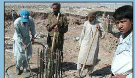
Shelter for Life International is helping rebuild roads, housing and schools in Afghanistan. Photo: Shelter FOR Life International
