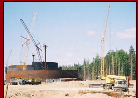
OPIC will provide $130 million in financing for the construction of an oil export terminal in northern Russia. Above, a tank farm is constructed at the project site in Vysotsk.
