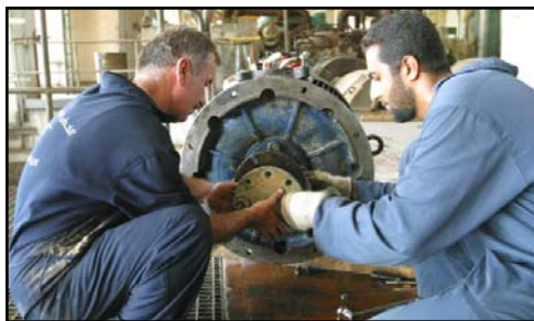
Iraqi workers renovate the Al-Doura power plant in Baghdad, with USAID support.
