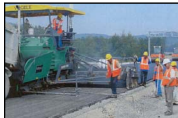
Construction of a viaduct at Modrus, top right, and new asphalt on the road to Split are all part of the Croatian Motorway project supported by OPIC insurance.
