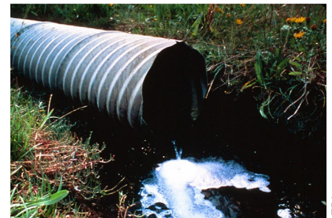
Discharge from pipe
