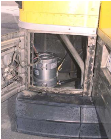
Figure 8. Close-up of filter system in rear engine compartment for a bus equipped with a Series 50 Detroit Diesel engine. The doors were installed to provide access space for the filter.
