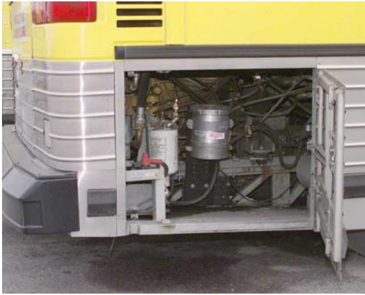
Figure 6. Photograph of Caterpillar engine filter system through side engine compartment door.
