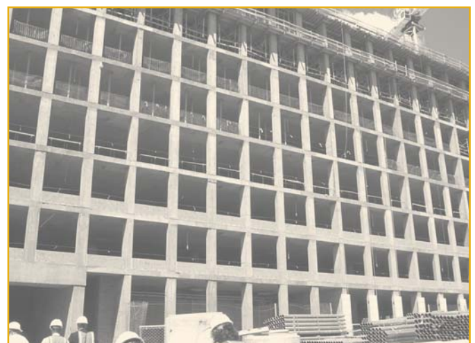
During construction its working title is "Building E," but USPTO will officially name this structure the Remsen Building. It is scheduled to be completed by the end of 2003.
