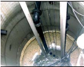
Sewer system component
